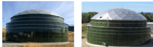
Africa GFS Anaerobic Digester Tanks
